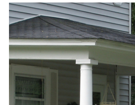
Prairie Trail examples showing a deep eave type and a boxed eave return
